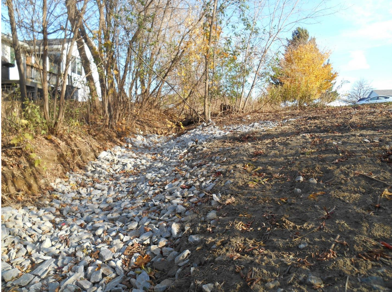
Figure 8: New stone cover in existing drainage swale, near location of proposed infiltration basin.
