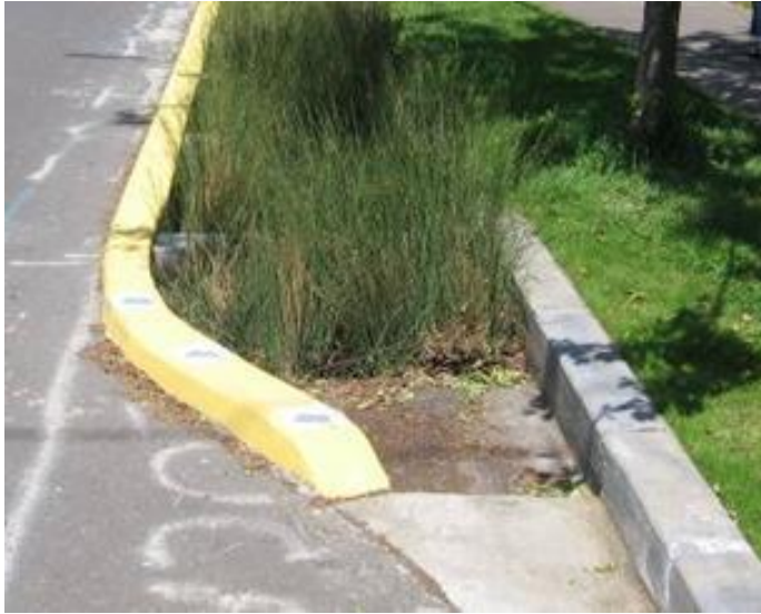
Figure 14: Example of a stormwater curb extension for the Route 7 ROW (Credit- VA DRC Stormwater Design Manual 2013).
