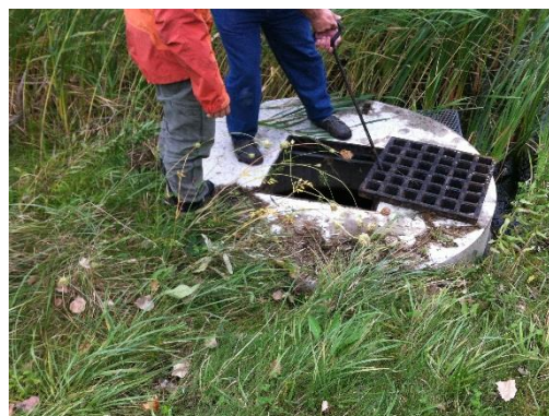
Figure 2: WCA and Town Public Works Director Inspect #3410-9010 Outlet structure to verify pond routing.
